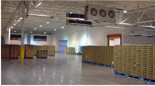
Figure 3. Strawberry cold storage room with unused space.
