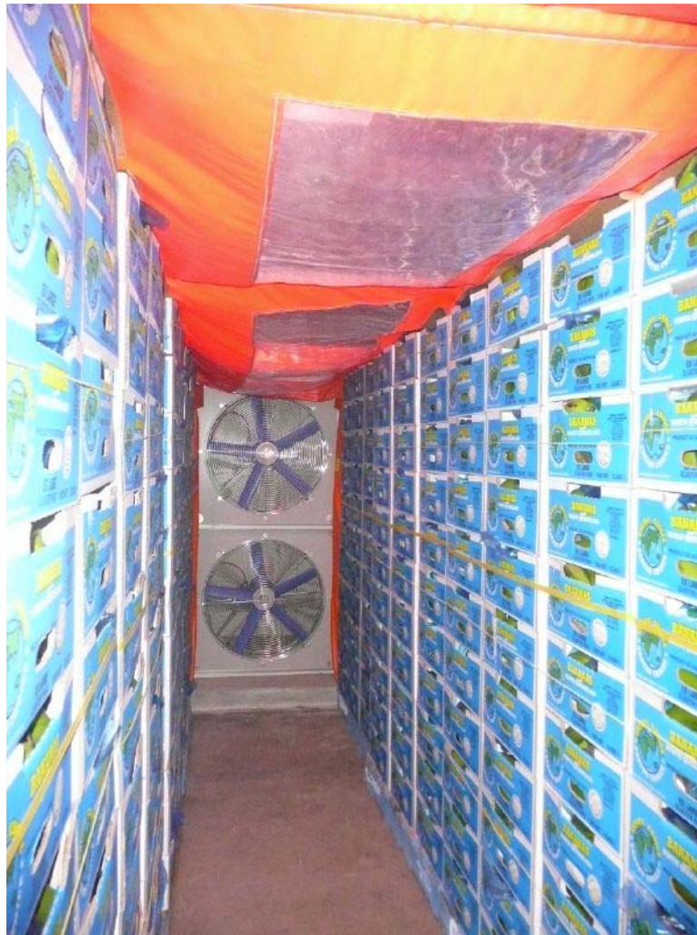
Illustration 1: Tarp Tunnel Precoolers are the Front-Line in Rapidly Cooling Fresh Produce
