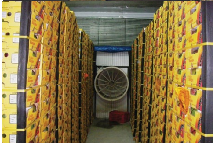
Forced-air cooling tunnels
